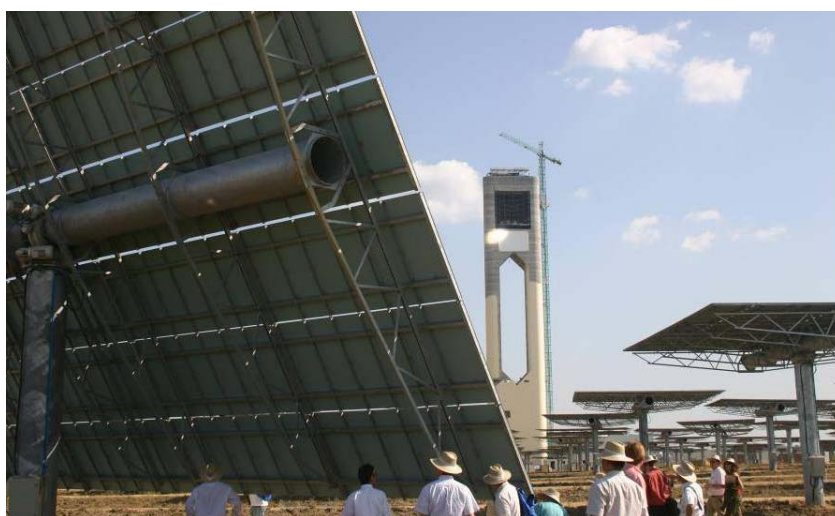
Figure 3 The PS10 central receiver solar thermal power plant under construction in Spain, June 2006.
